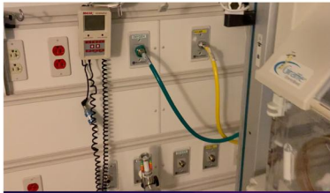
e) Space for infusion pumps and O 2 in a NICU room
